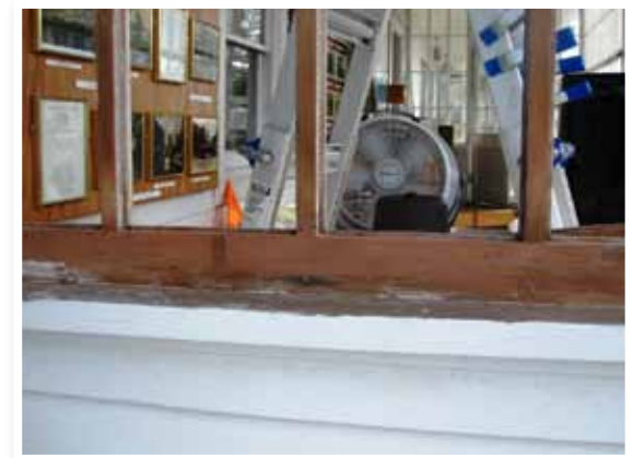
Top photo: A close-up of the sunroom window framing on July 8 demonstrates the degree of damage and wood rot sustained by the redwood material.
