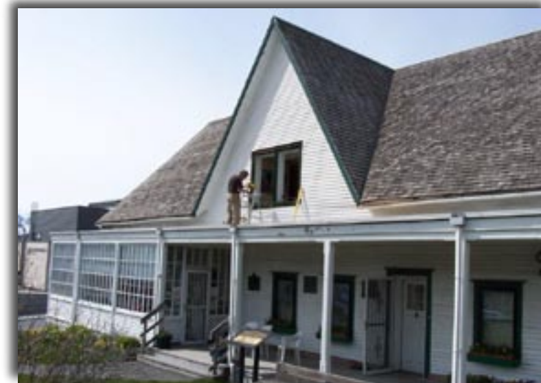
Historic mill work specialist Don Corwin from Skagway, Alaska, examines the signature gable window on the Baranov Museum. A man of many talents, Don will also be on the salmon grill at our Praznik on Sunday, August 3rd. Stop by to say hello to Don!
